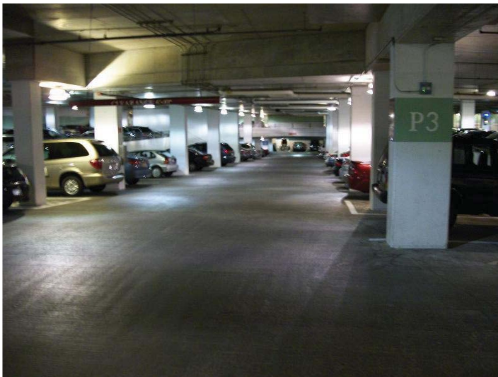
General Layout with ramp in the middle and parking on both sides and at the other end.
